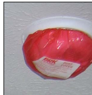
Smoke detector in HUD unit
