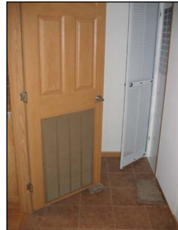
Return air grill in utility room door
