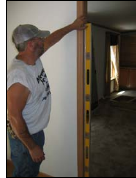
French door opening out of plumb
