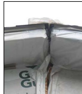
Gap remaining at ridge
