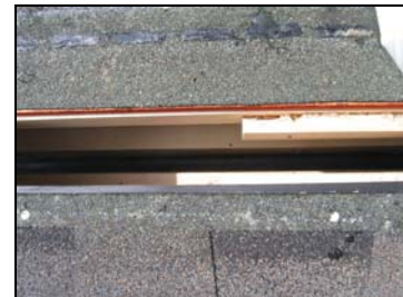
Gap at ridge
